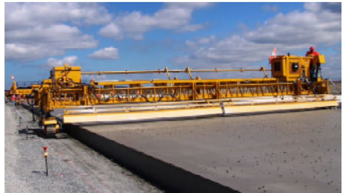
Sea-Tac's third runway is 17-inches thick and is created by using a slip-form paving machine.
